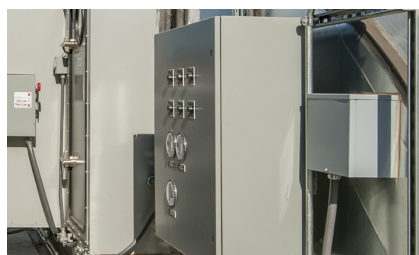
Rooftop Control Systems
