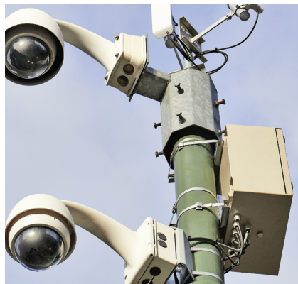
Surveillance and CCTV Systems
